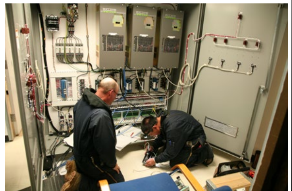
Figure 2 - The motor control cabinet being wired and tested in the old LAMA room.
