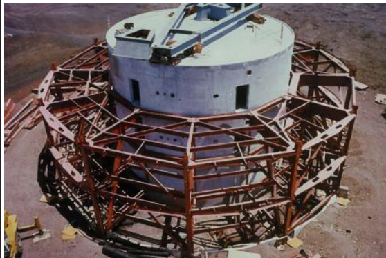
The pier is seen during construction with the base (A-frame) of the telescope already installed at its top. The metallic structure being erected around will ultimately support the dome.
