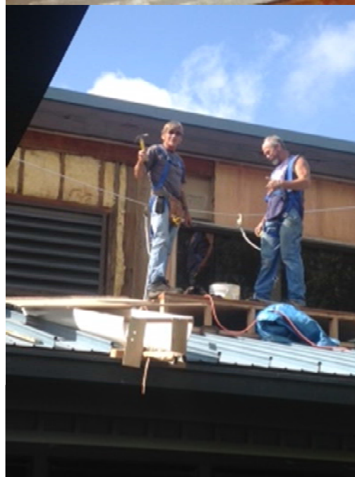
Figure 26 – Top: The front lobby of the office underwent a large upgrade with the addition of new wooden flooring, a custom 3D rendering of the CFHT logo, and new furniture to greet our guests. Bottom, Roger Wood and Joe Fehly work on replacing aging exterior panels on the office.
