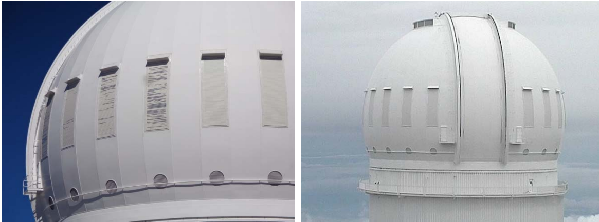
Figure 15 – New dome vents suffered premature paint peeling (left) under high wind conditions. Working closely with the manufacturer this was addressed through the installation of replacement vent slats (right). Extensive environmental testing of the new slats gives confidence that they will weather much longer than the original ones.
