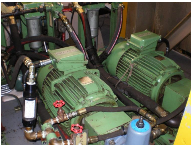
Figure 21 - Telescope hydraulic pump station showing the location of the transfer hose.
