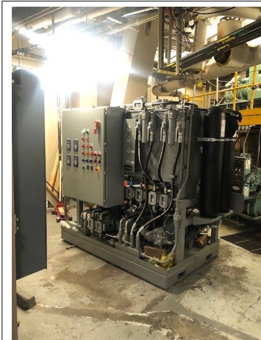
New Hydraulic Power unit installed at the summit.
